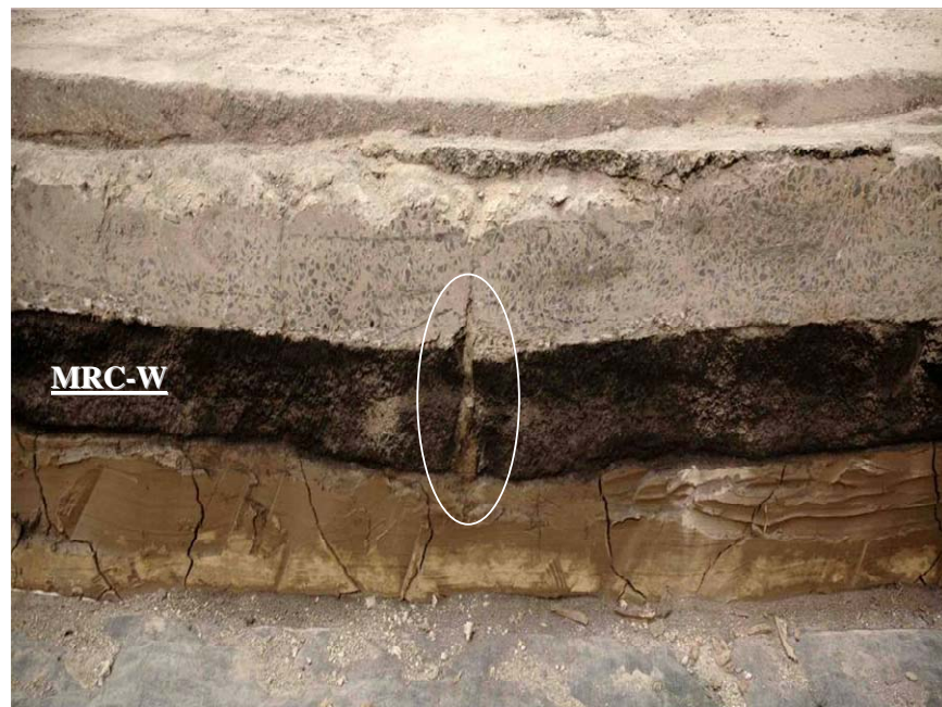
CLOSE-UP OF MRC FAILURE
